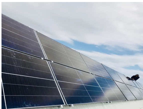
Steve Cornthwaite of Micro Energy Systems installed SEWACS' new 6.3kW three phase solar system
